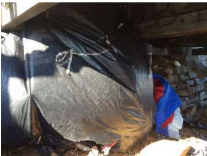
Figure 29. Illegal occupation under the Wooden Bridge.
