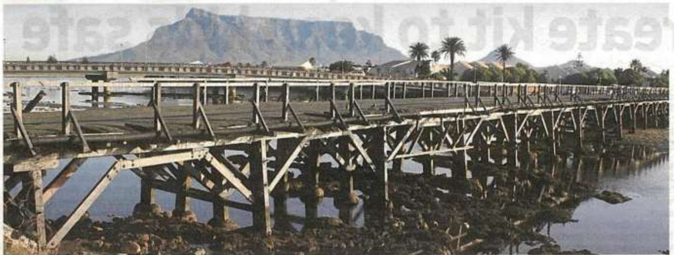
Concerns over the derelict wooden bridge across Milnerton Lagoon have been raised.
